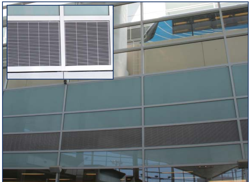
Figure 4: View of wide CT diffusers set into the window framing that is installed above the ticketing counters and along the walls of the inside security area. (Inset is a close-up view of the wide CT diffuser.)
