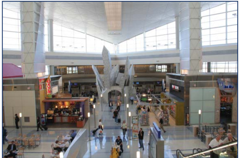
Figure 2: Sections of special CT diffusers located in one of the two terminal building concession areas. Note the modular style of the architecture.
